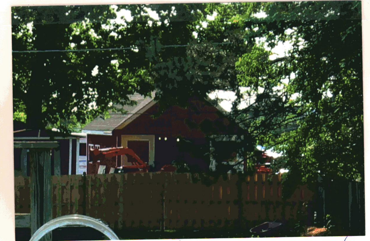
Constant heavy equipment use, to move gravel & soil (regrading) around. After easement was complete
