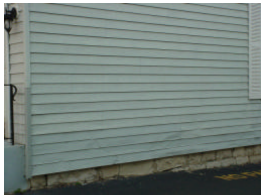
Fig. 36: Vinyl and aluminum siding are discouraged materials and should not be used to cover historic building materials
