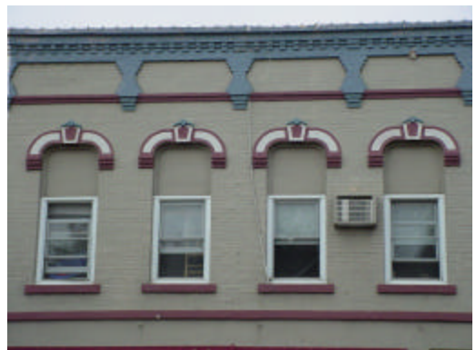
Fig. 29 Replacement windows should fill the entire historic opening. Avoid replacing windows where the window opening is not filled
