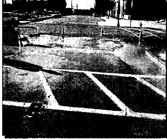
Leak surfacing at intersection
