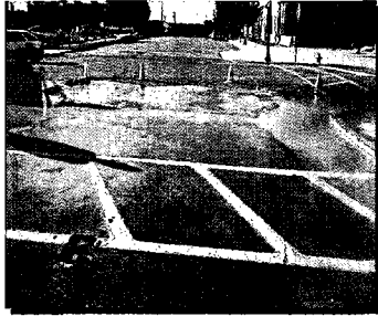
Leak surfacing at intersection
