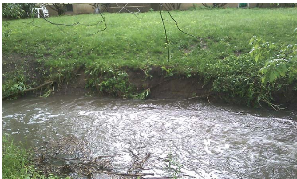
Erosion at Bend Near House
