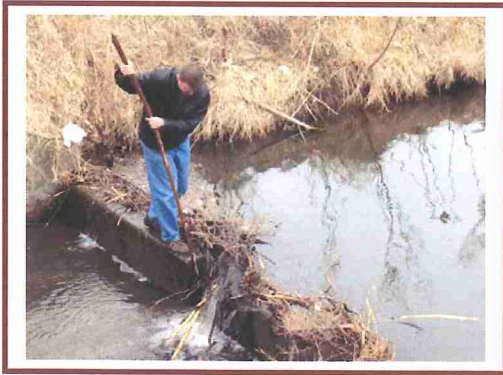
Figure 1: Dam with debris blocking notched concrete
