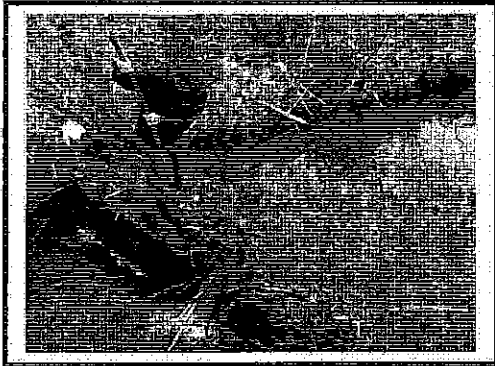
Figure 1: Dam with debris blocking notched concrete
