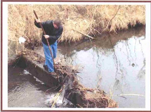
Figure 1: Dam with debris blocking notched concrete
