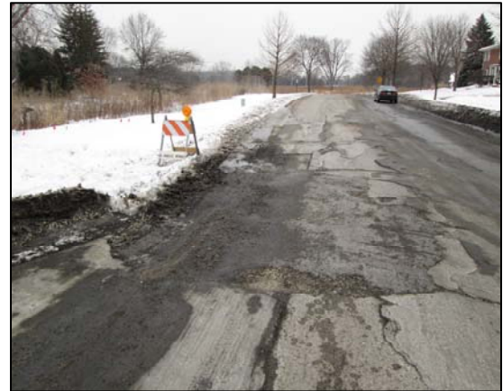
Figure 1-1. Pavement Deterioration. Pavement throughout the Orchard Brook East Subdivision has suffered significant pavement deterioration. This can be seen throughout the project area.
