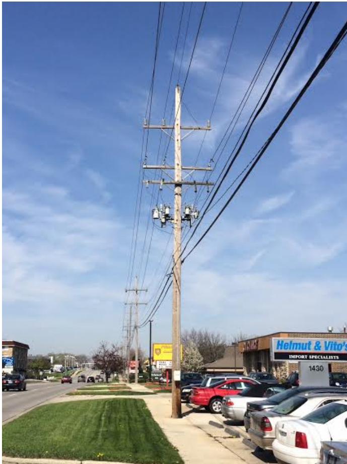
Utility lines on commercial property west on Ogden Avenue
