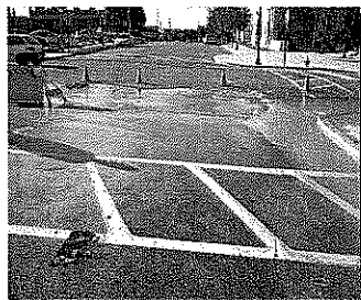
Leak surfacing at intersection
