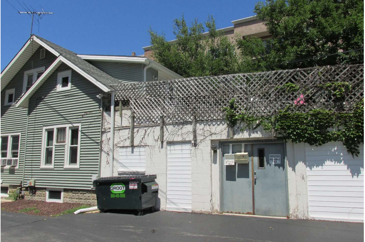
Figure 3 - Photo shows the south elevation of the subject building. The second floor of the subject building currently houses a vacant apartment.
