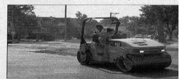
TOP COAT: A steamroller flattens the asphalt down on Thursday on Grand Boulevard in Brookfield.
