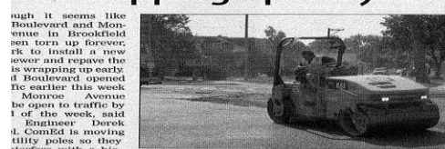
TOP COAT: A steamroller flattens the asphalt down on Thursday on Grand Boulevard in Brookfield.
