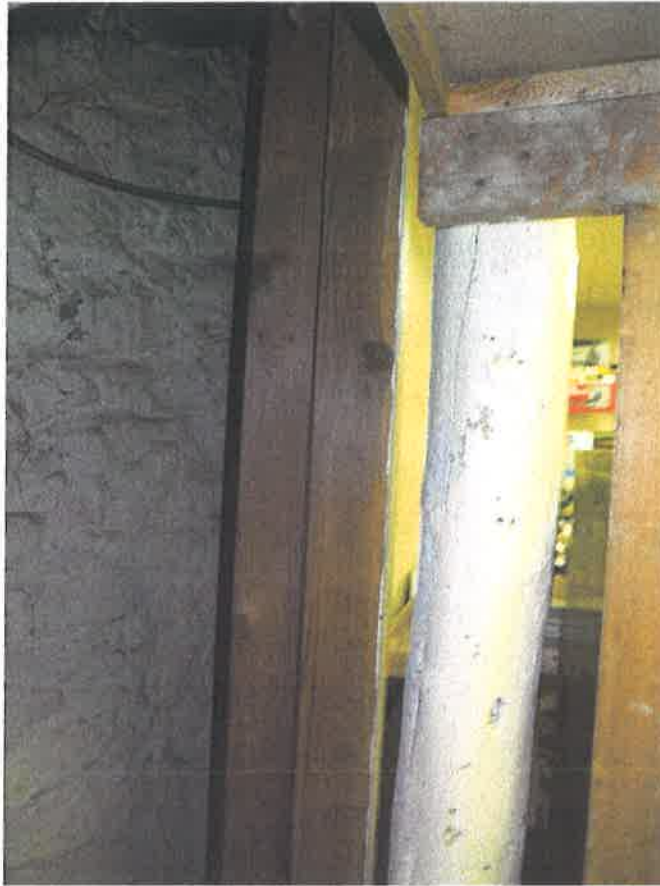
Photo #9: View of the log/tree trunk support for the main beam running east to west under the house (2016)
