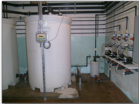
Liquid Chlorine installation at an existing pumping station
