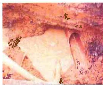
Hidden leak running into drain tile
