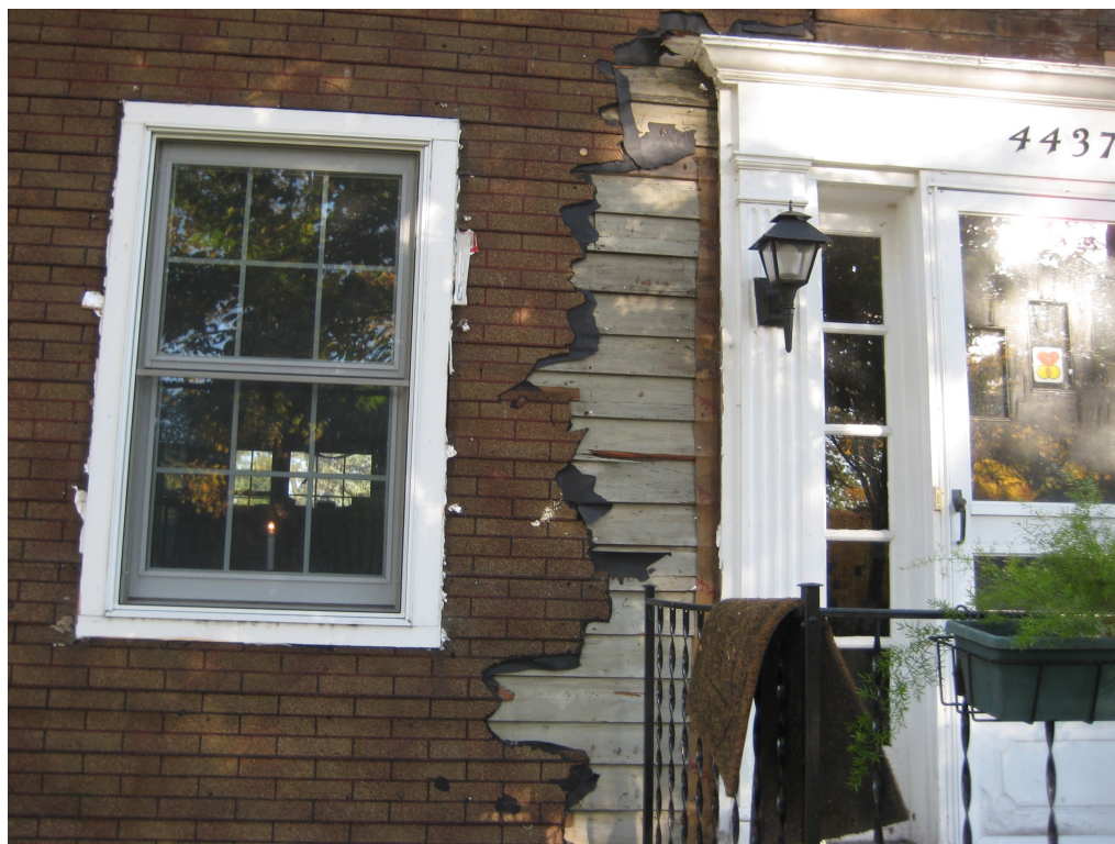
Close up showing original clapboard covered with 1930's brown, fake-brick tar paper after aluminum siding removed (photographed during 2008 exterior residing project)
