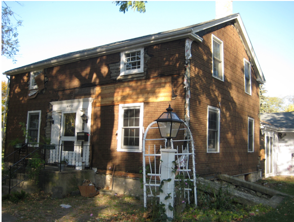
House after removal of 1960's vintage 8-inch aluminum siding and prior to installation of 4-inch fiber-cement siding (photographed during 2008 exterior residing project)
