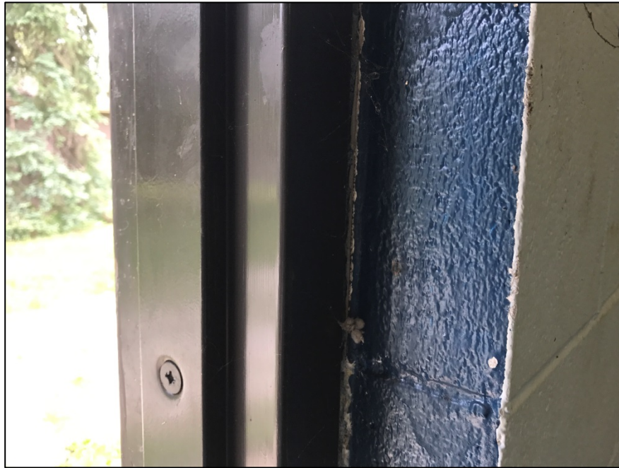
Photograph 3 – A view of the asbestos containing beige interior door caulk.
