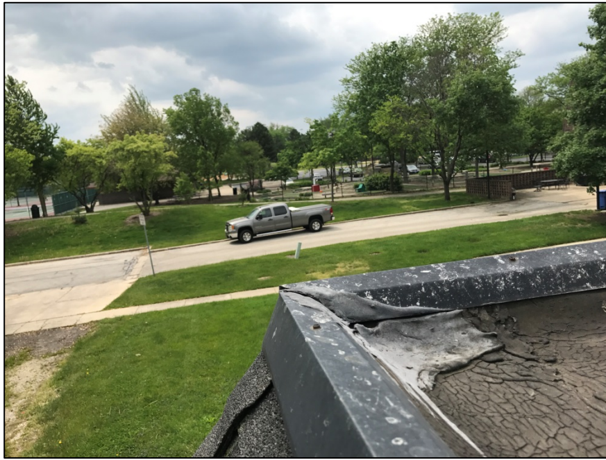
Photograph 5 – A view of the asbestos containing black roof tar patch on the roof.
