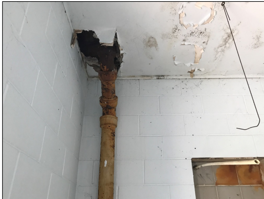
Photograph 6 – A view of the interior of the building showing the drywall ceiling and the asbestos containing drywall compound.
