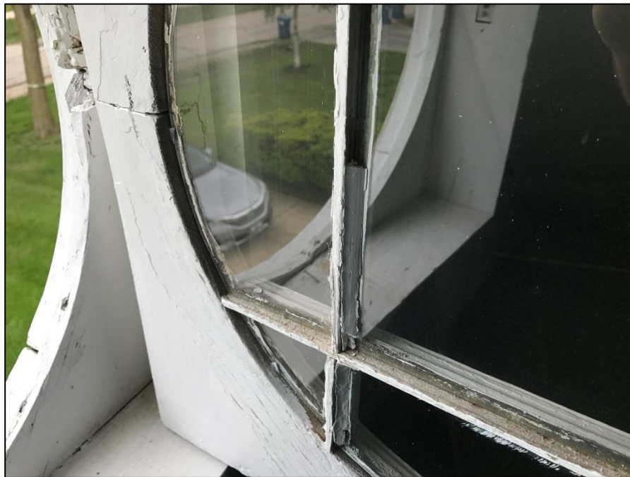
Photograph 4 – A view of the white window glazing on the small 2 nd floor front attic window.
