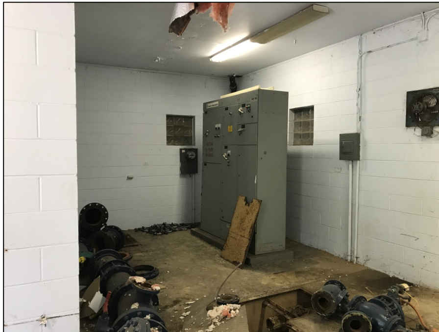
Photograph 2 – A view of the interior of the building showing the drywall ceiling and the asbestos containing drywall compound.
