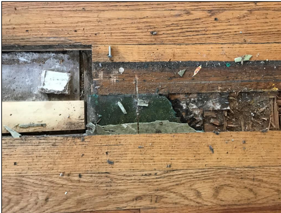
Photograph 2 – A view of the green and light green flooring under the wood floor in the kitchen. The light green flooring is asbestos containing.
