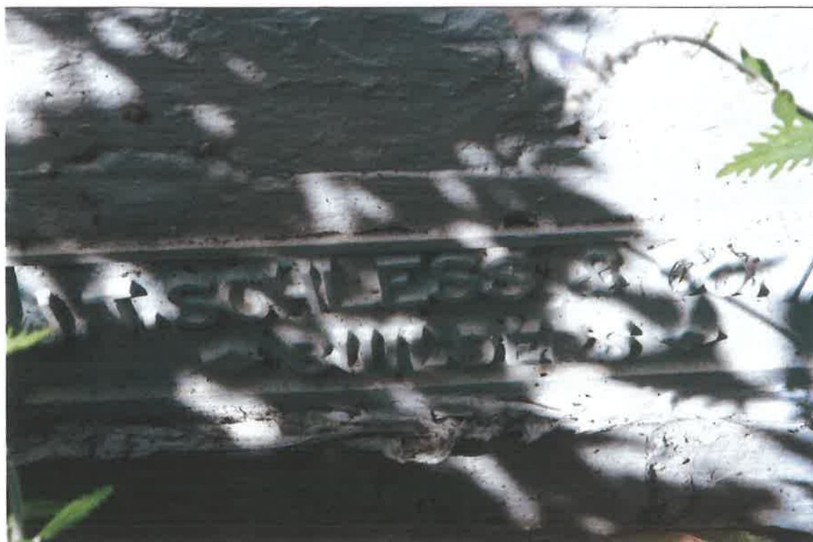
Photo #4: J.T. Schless Co plate on foundation Oct 5, 2017
