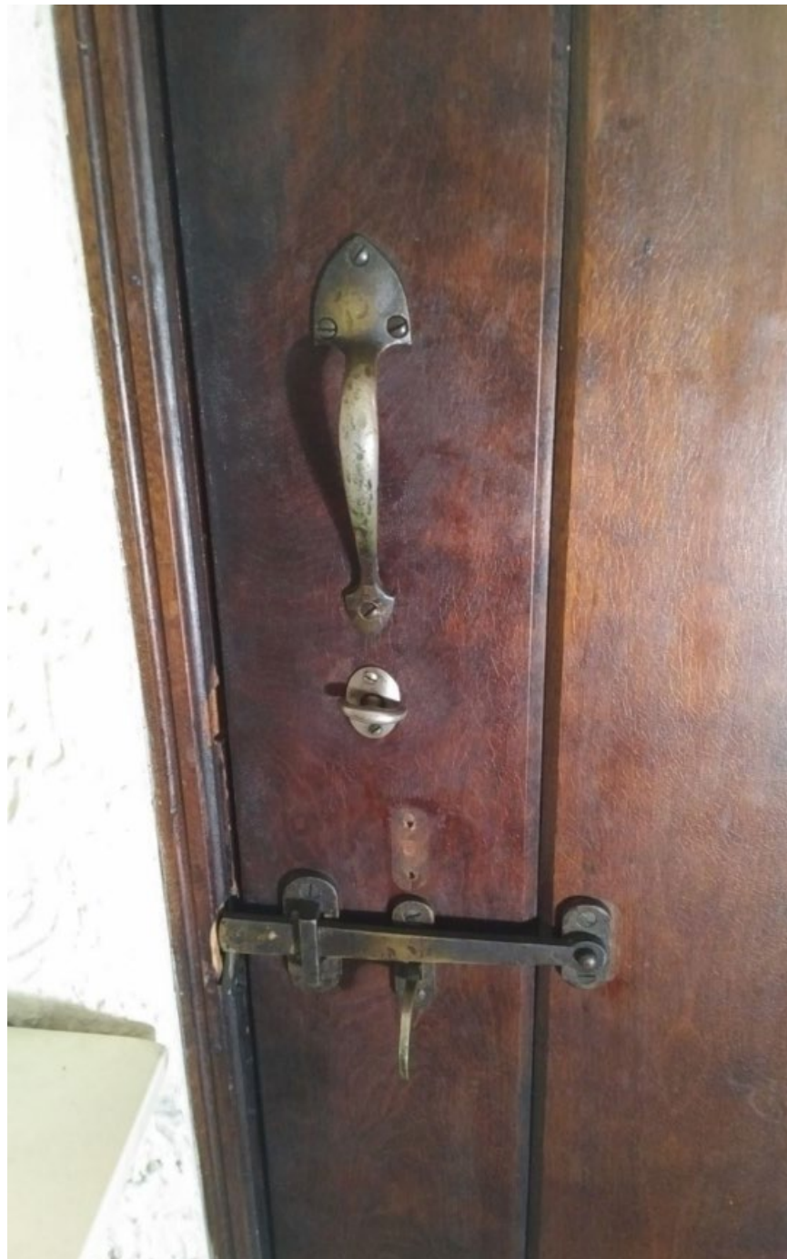
Figure 13 – Period Door Hardware
