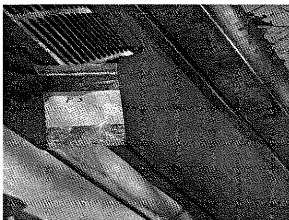
Photo 3 – View of white paint on exterior wood soffit.
