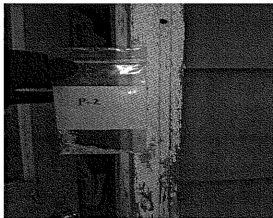
Photo 2 – View of white paint on wood door frame.
