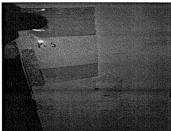
View 5 – View of white paint on drywall wall.
