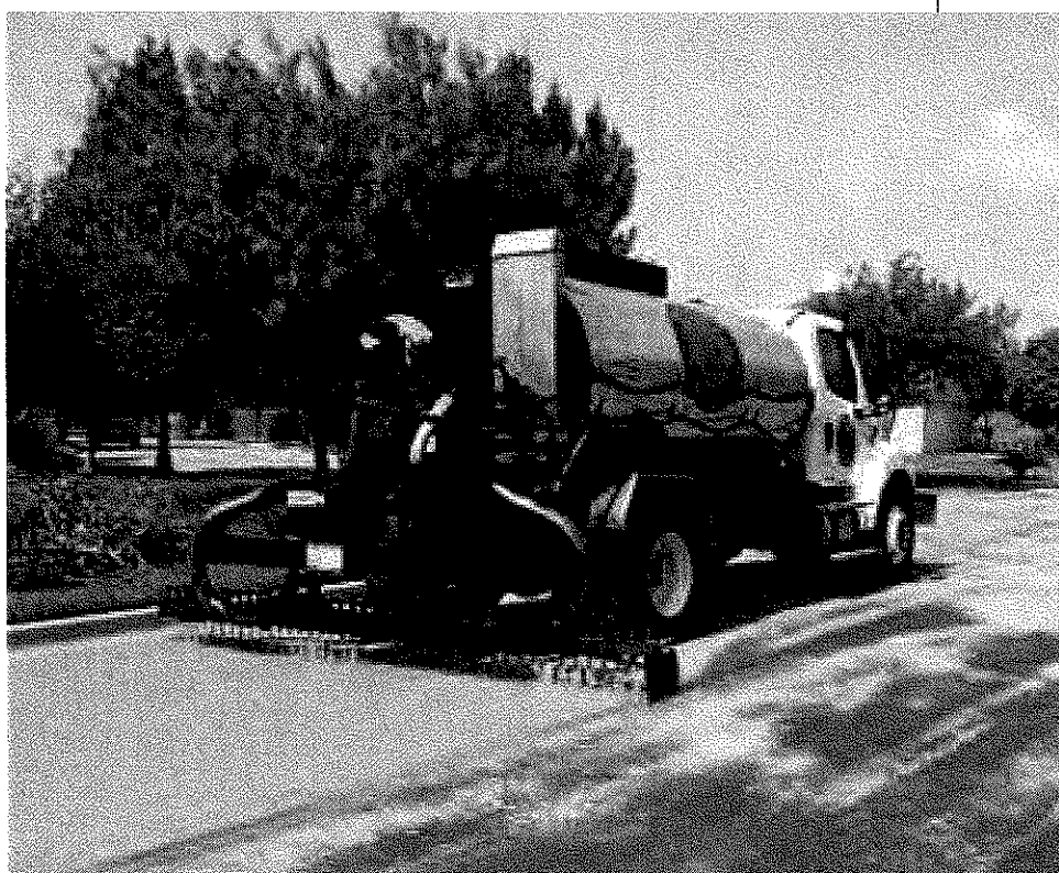
Pavement Restoration, Inc., Boerne, Tex., applies Reclamite rejuvenator to pavement in Travis County, Tex.
