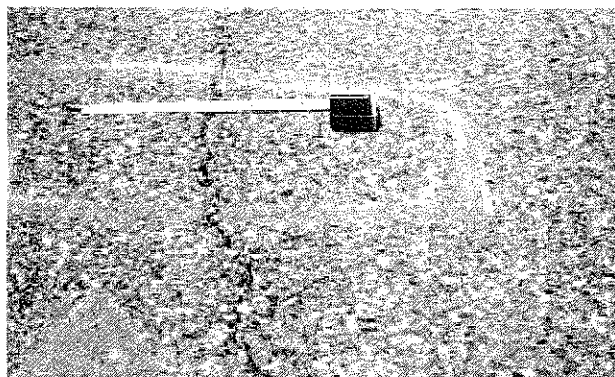
April, 1970—Age 36 Months. South Transverse Crack.
