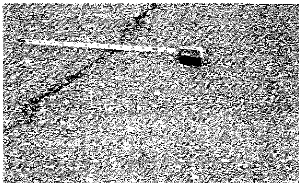
April, 1969—Age 24 Months. North Transverse Crack.
