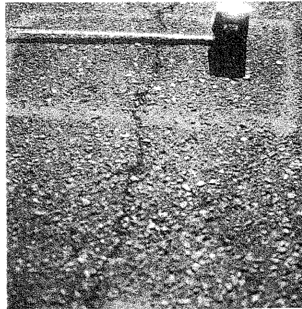
August, 1970—15 Months after Reclamite.
