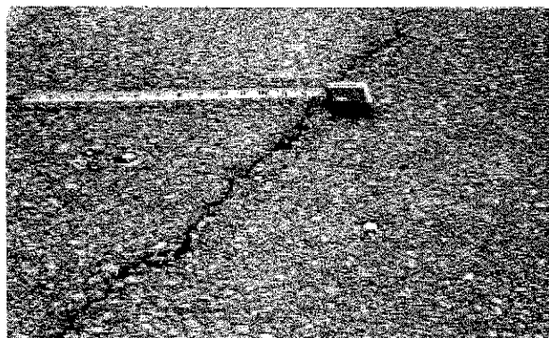
April, 1969—Age 24 Months. North Transverse Crack.
