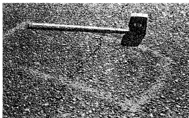
August, 1970—15 Months after Reclamite. South Transverse Crack.
