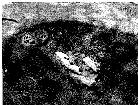
Correcting and replacing old and obsolete infrastructure will be a core part of this project, including this inlet and connecting pipe at Dawn Place and Stanley Avenue.
