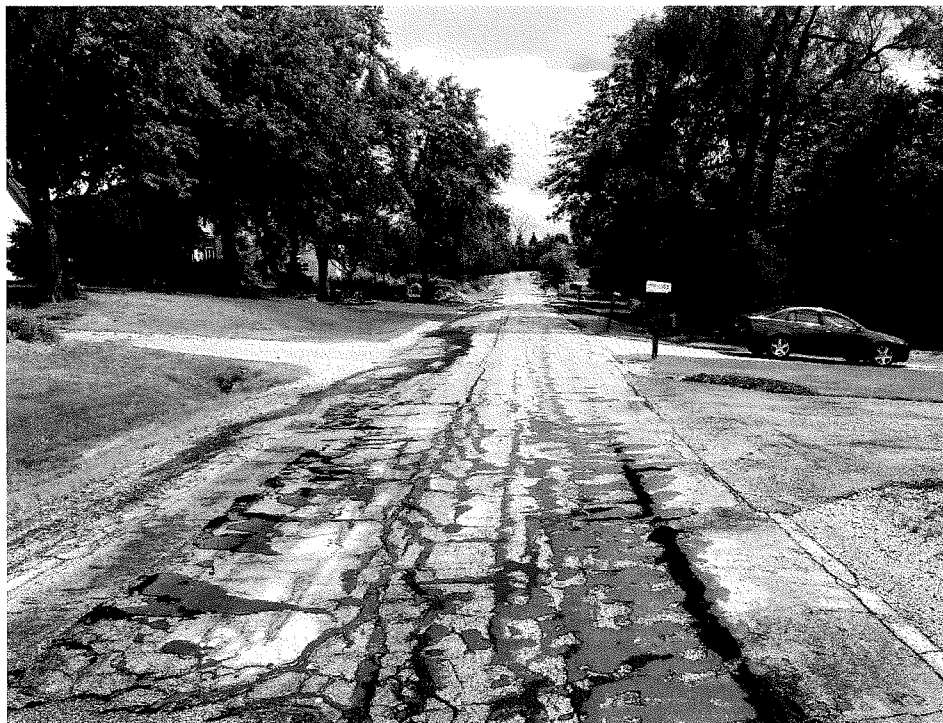
Cross Street looking south. The existing roadway is in poor condition, and requires resurfacing. Erosion control will be important given grades along the project corridor and installation of sidewalk in western ROW.
