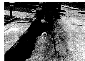
We are familiar with sewer and roadway resurfacing construction methods, and construction observation requirements.
