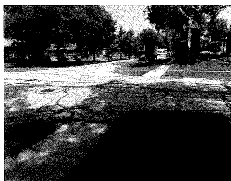
Correcting detectable warnings and improving pedestrian access will be addressed at intersections and road way approaches, including areas such as Sherman Street and Stanley Avenue.
