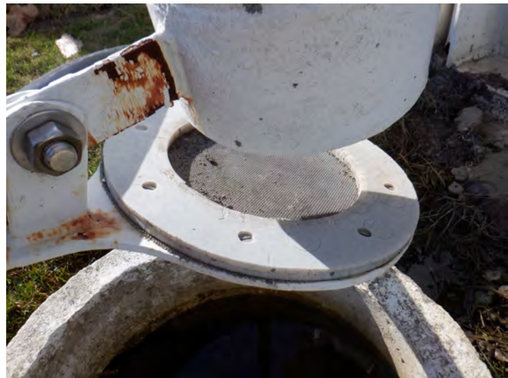
17) The screened flap gate on the overflow pipe is in good condition.
