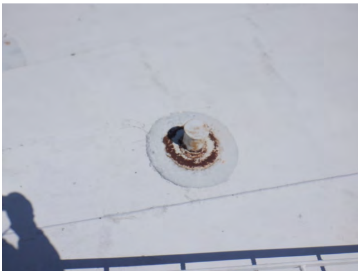
33) Coating failures at a roof rigging coupling.
