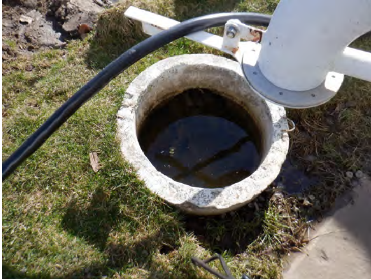
16) The overflow discharge is not in line with the catch basin.
