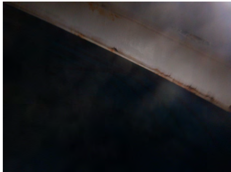
44) Corrosion on the edge of a roof stiffener.
