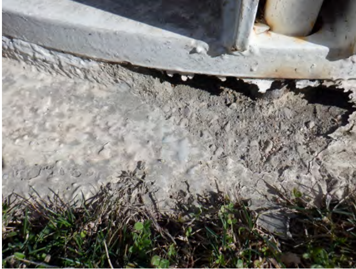
10) Missing grout between the baseplate and foundation on a leg.
