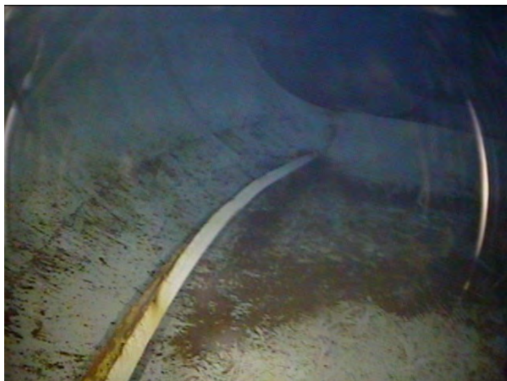
52) A piece of the sidewall stiffener/painter's railing on the floor of the tank.
