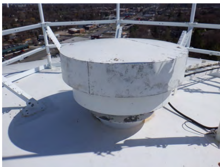
35) Coating failures on the roof vent.
