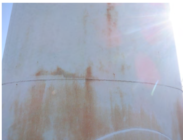
5) Coating failures on the riser.
