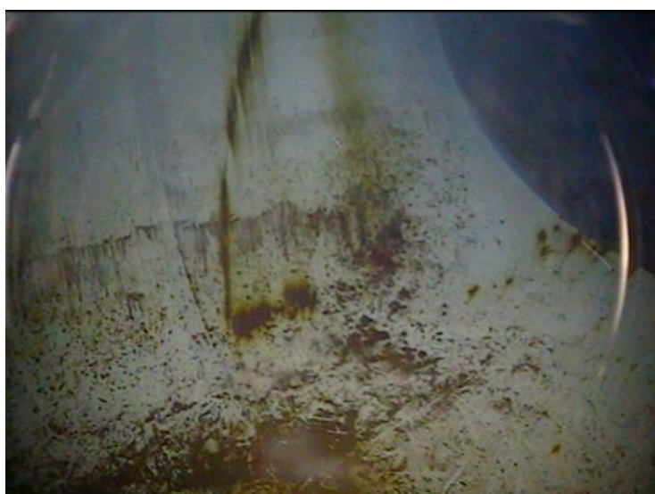
51) Coating failures on the bowl.
