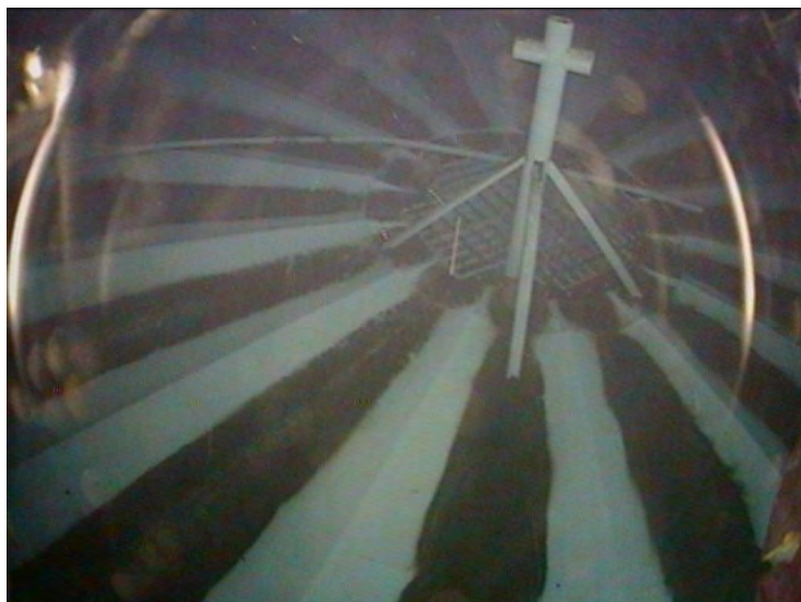
49) Sediment on the wet interior bowl.
