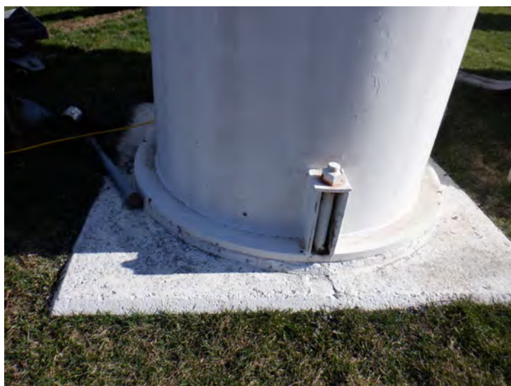
9) The leg foundations are in good condition overall. The anchor bolts are in good condition.
