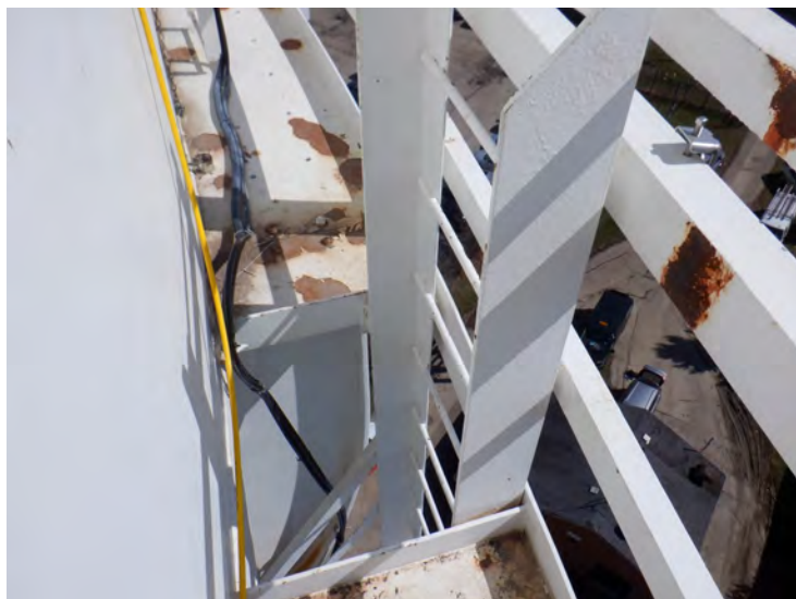
22) There is a ladder opening in the balcony. There are chains on either side of the opening. There is no fall prevention device on the ladder from the stairs to the balcony.
