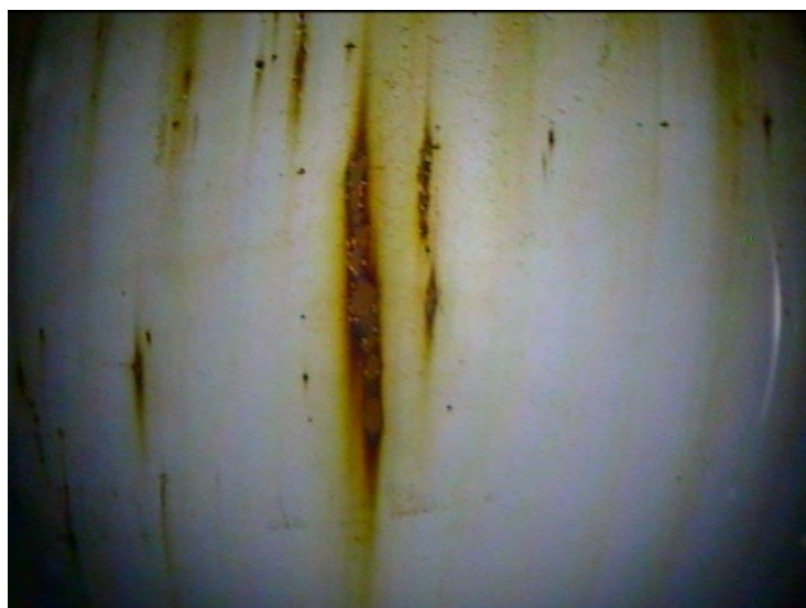
45) Coating failures on the wet interior sidewall.
