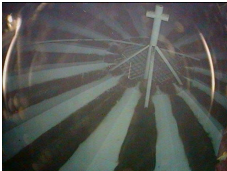
49) Sediment on the wet interior bowl.
