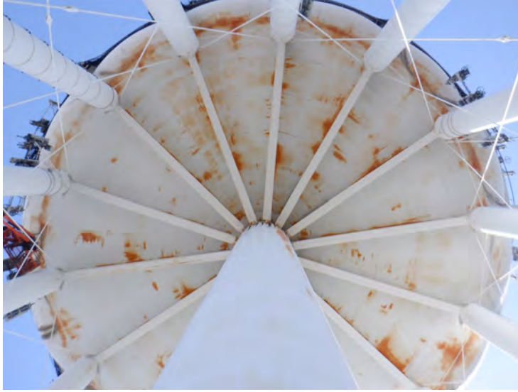
19) Coating failures on the bowl.
