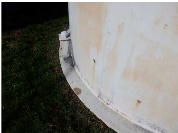
1) The riser foundation is covered with soil and not visible for inspection.
