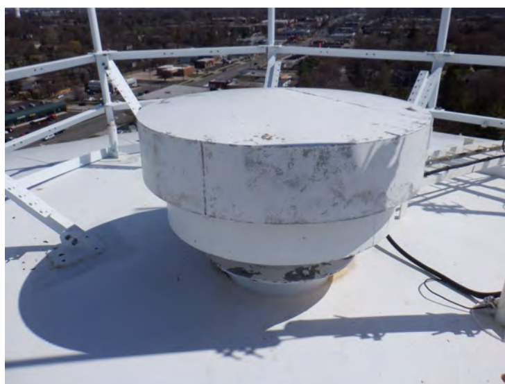
35) Coating failures on the roof vent.
