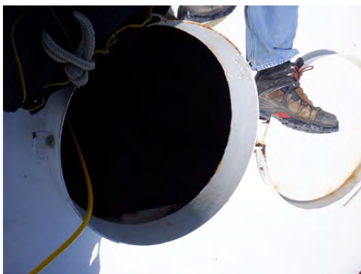
39) There is no gasket on the wet interior roof hatch.
