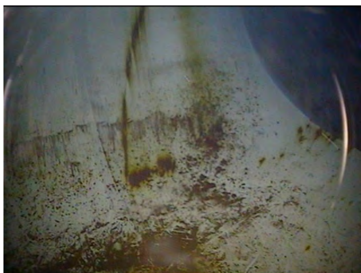
51) Coating failures on the bowl.
