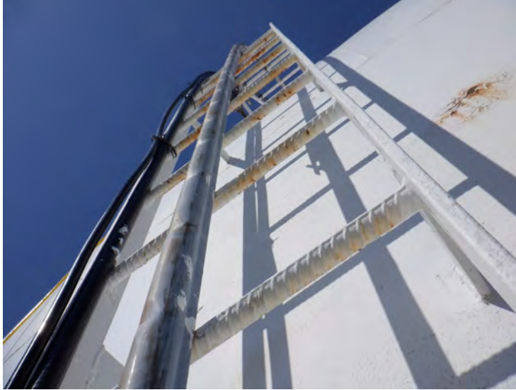
28) The sidewall ladder is in good condition. The fall prevention device is in good condition. Antenna cables are attached to the ladder and interfere with climbing.
