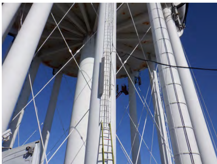
18) There is no longer a vandal guard on the leg ladder. The ladder and fall prevention device are in good condition.
