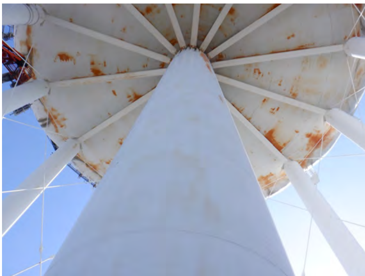
6) The riser coating is in poor condition overall.
