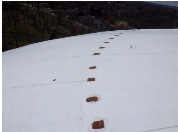
32) Coating failures on the roof.
