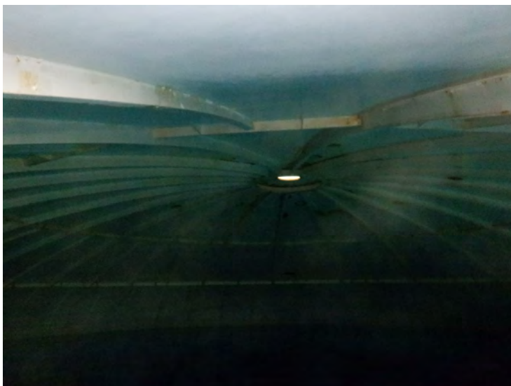
42) Coating failures on the wet interior roof.
