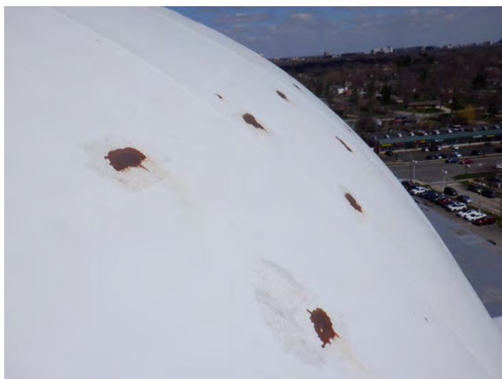
30) Coating failures on the roof knuckle.
