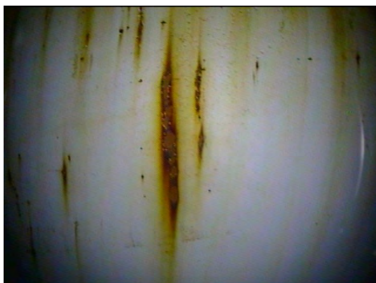
45) Coating failures on the wet interior sidewall.
