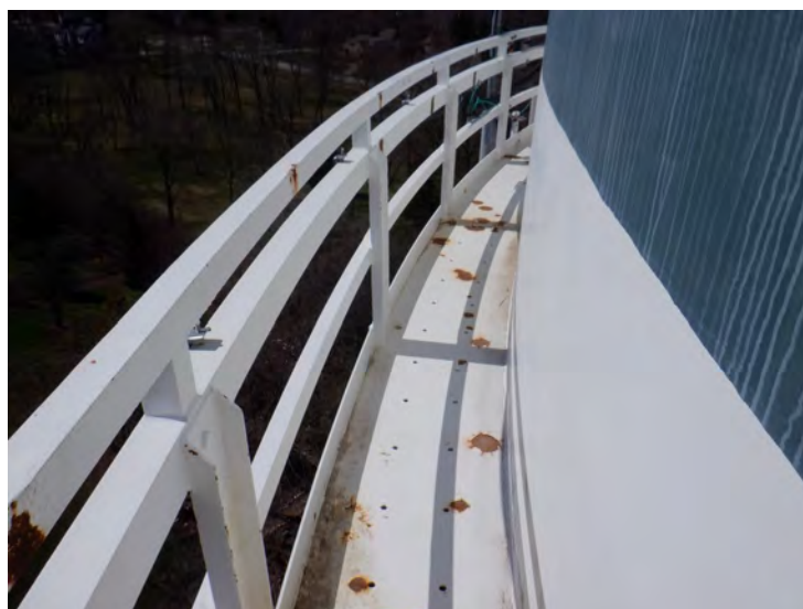
23) The balcony coating is in poor condition.
