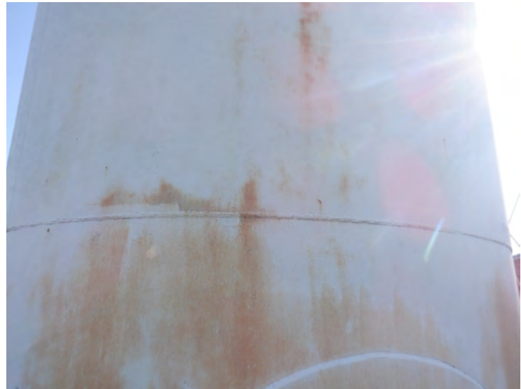
5) Coating failures on the riser.
