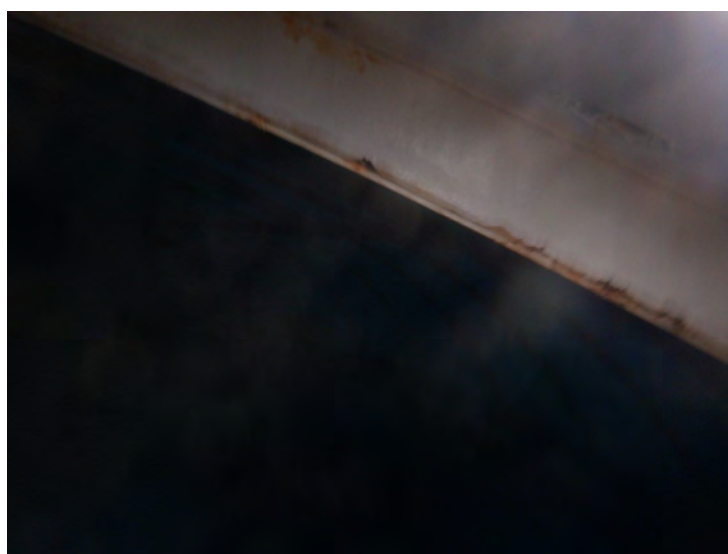
44) Corrosion on the edge of a roof stiffener.
