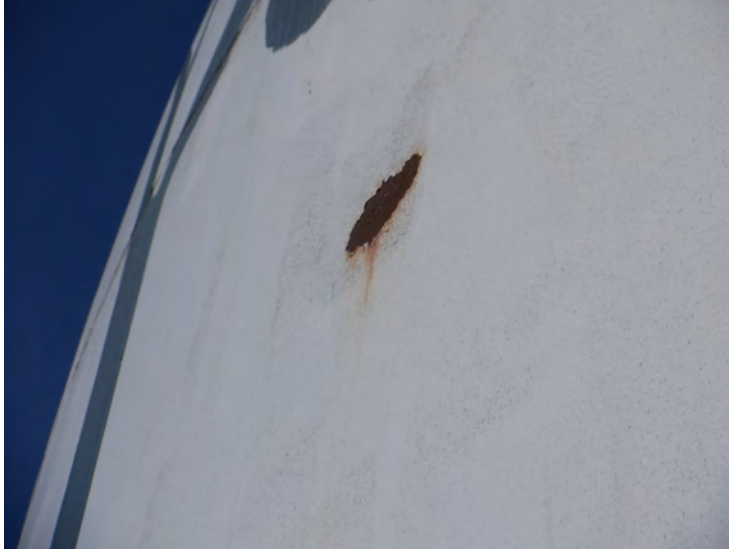
25) Coating failure on the sidewall.
