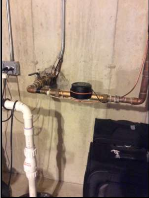
Completed Installation Photo
