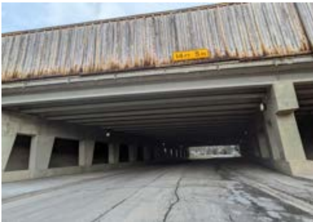
Underpass conditions at Jackson Drive and I-355 leading into Downers Grove. There is minimal lighting and pavement is damaged due to run-off
