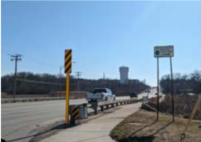
A narrow bridge next to 40 mile per hour traffic at Highland Avenue and 35th Street
