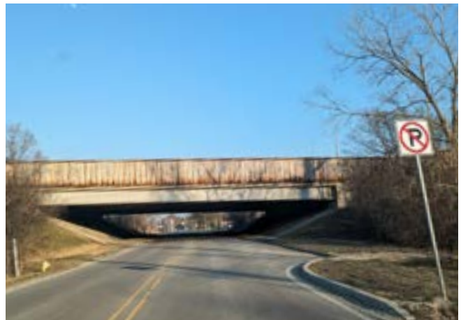
Underpass conditions at Hitchcock Avenue and I-355. There are no continuous sidewalks or bridge lighting. Utilities are adjacent to the road edge and debris was observed along the pavement edge.
